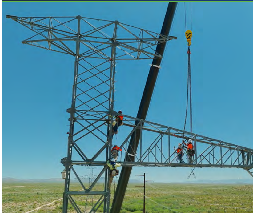
Transmission tower construction for the SunZia Wind power project. Photo credit: Pattern Energy
